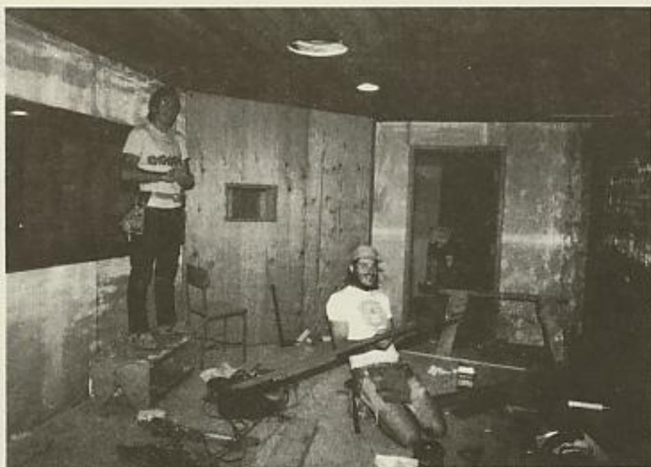
Ron Craig and Mike Harman apply redwood paneling to the walls of the audio control room.
