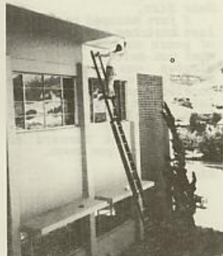
Tery McCade puts the finishing touches of paint on the building's exterior.
